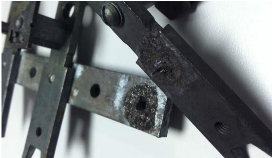
This is a failed, high-resistance, busbar connection inside a 200 ampere Stab-Lok panel. The arced-away steel screw holds the copper bar in the forefront to the aluminum bar in the background.
